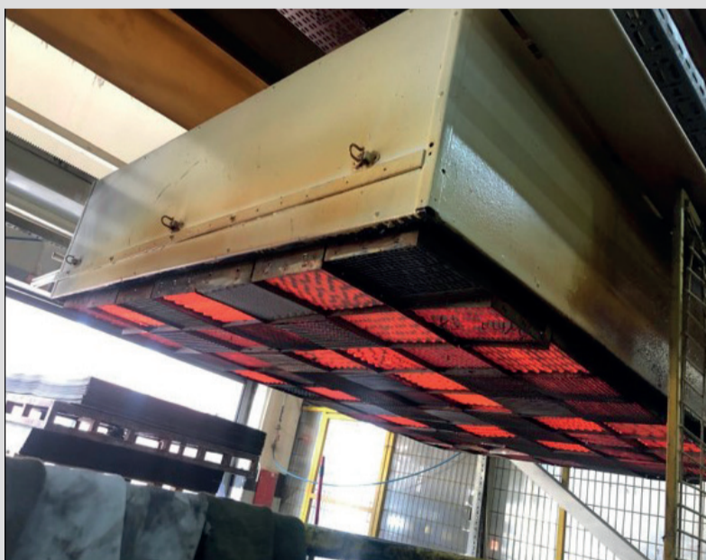
Inefficient combustion due to phase imbalance.
